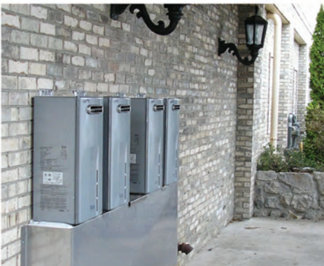
Full service restaurant gains extra mechanical room square footage for additional storage plus redundancy by installing multiple units on the exterior wall.
